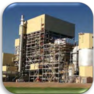
Utility Steam Generation
