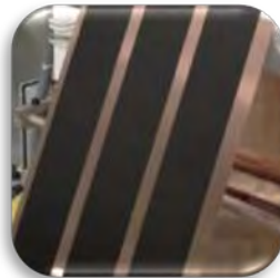
Coating and Drying Equipment
